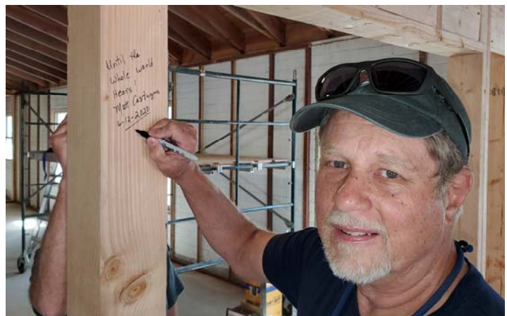
Before leaving IBC, we prayed for the facility and wrote verses on parts of the wall which will be covered with sheet rock.
